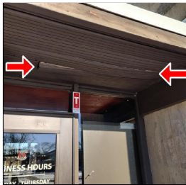
1.3 Item 1(Picture) Wood soffit is damaged, wood is bowing
