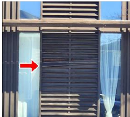
1.3 Item 3(Picture) A siding panel is detached from the wall
