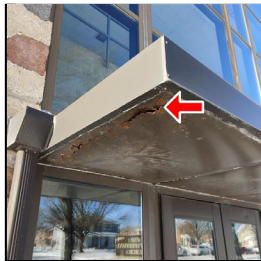
1.3 Item 2(Picture) Soffit panels are rusted at the north building main entrance
