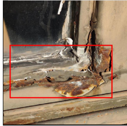
1.4 Item 2(Picture) A view of sill damage at middle building window
