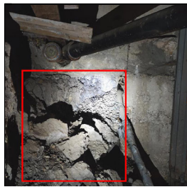
5.1 Item 1(Picture) Dirt and concrete id observed out of place creating the void in the background
