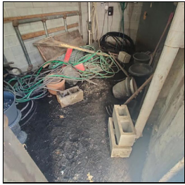
5.1 Item 2(Picture) A view of the dirt covering the floor at the basement storage room at south building
