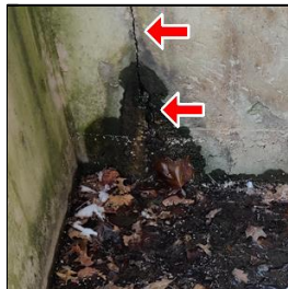
5.3 Item 1(Picture) Running water was observed at this crack
