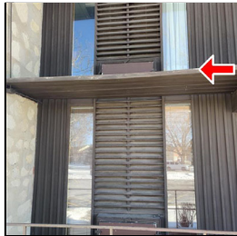
1.3 Item 4(Picture) Decorative eaves are bowed
