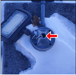
1.7 Item 1(Picture) Exposed wiring at damaged ground spot light fixture
