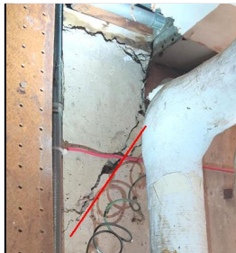
5.3 Item 3(Picture) A view of the same crack at the interior storage room
