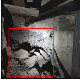
5.1 Item 1(Picture) Dirt and concrete id observed out of place creating the void in the background
