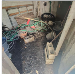
5.1 Item 2(Picture) A view of the dirt covering the floor at the basement storage room at south building
