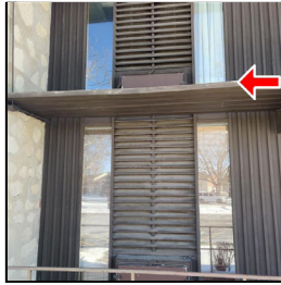
1.3 Item 4(Picture) Decorative eaves are bowed
