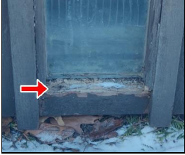
1.4 Item 1(Picture) Wood sill is damaged at south building
