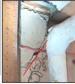
5.3 Item 3(Picture) A view of the same crack at the interior storage room
