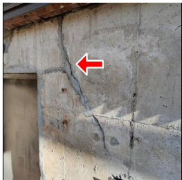
5.3 Item 2(Picture) A view of the failed crack repair at the basement foundation wall
