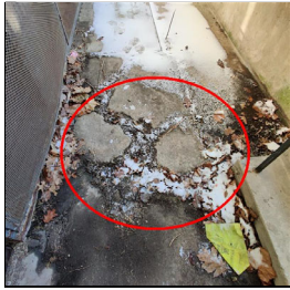
1.1 Item 1(Picture) Damaged concrete at the retaining wall walkway
