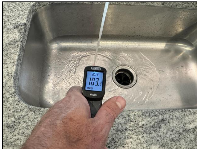
Hot water temp pool hose is a bit low. Recommend contractor increase temperature at water heater as needed.
