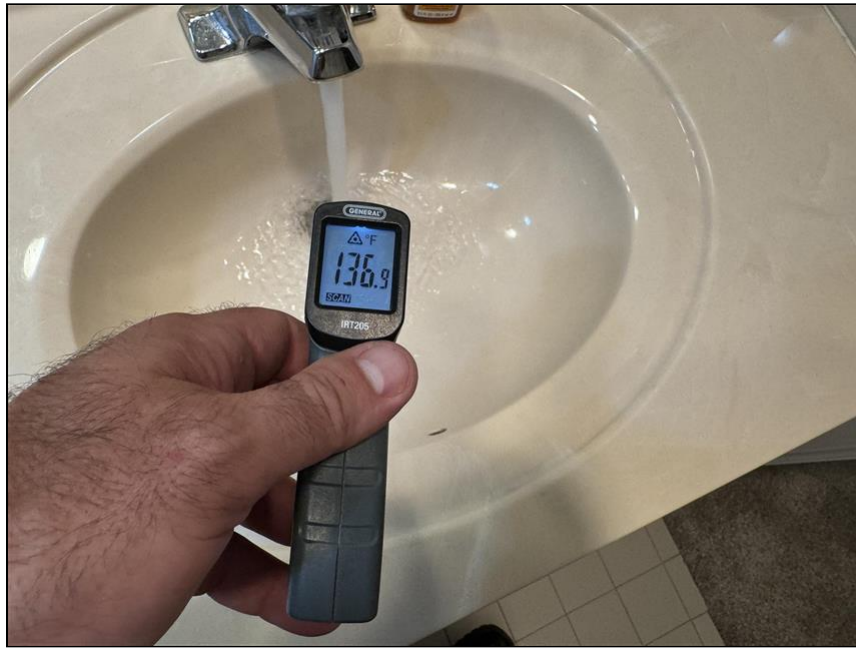
Hot water temperature main house
