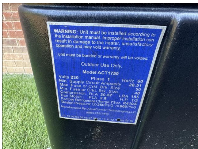
Pool heater data plate
