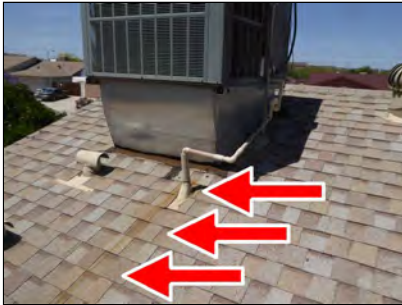
Unit 2 - Condensation Leak
