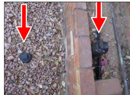
Main Plumbing Clean Outs
