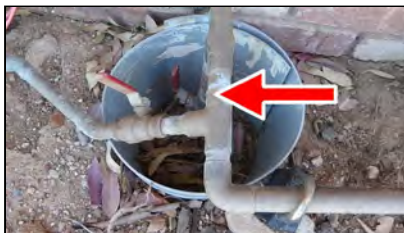
Main Water Shut Off Valve
