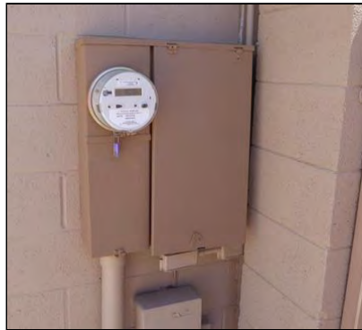
Main Electrical Panel
