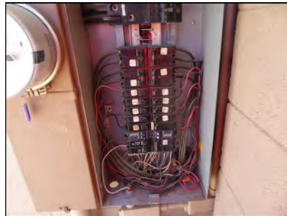
Main electrical panel with dead front removed
