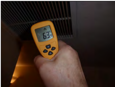
Unit 1 - Return Air Temp
